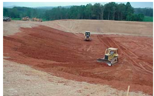
Figure 10D–11 Bathtub construction of clay liner (photo courtesy of NRCS Virginia (top) and NRCS Nebraska (bottom))
